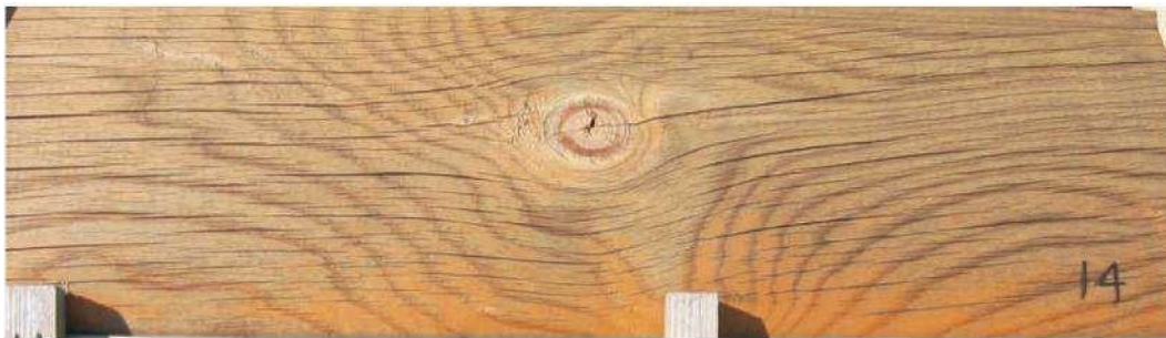
Fissuring of Log Siding
